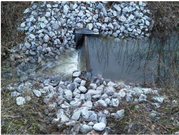
Figure B8-3. A water control structure.
