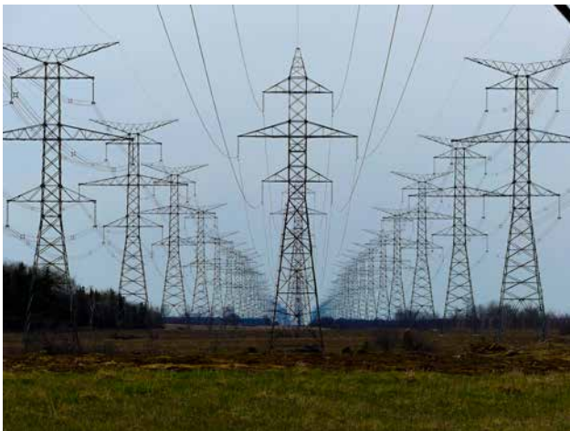
Figure C10–1. Large electricity transmission towers.
