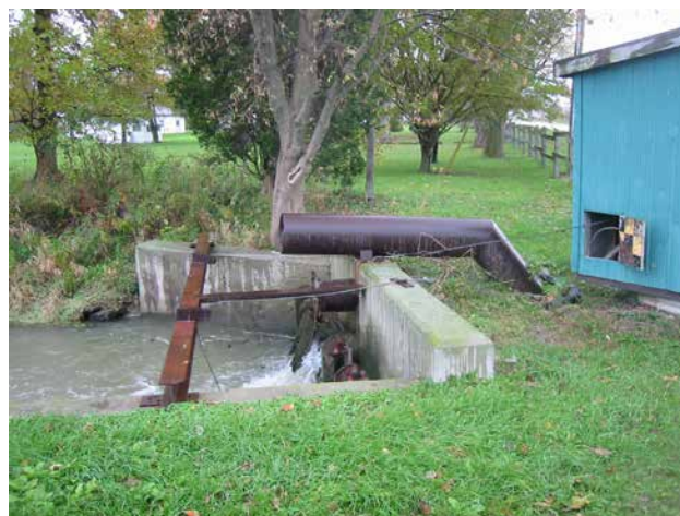
Figure B10-26. A pumping station.
