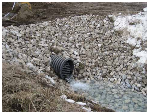
Figure B10-15. A drainage outlet.
