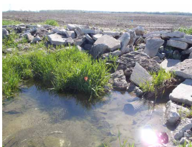
Figure B2–3. Example of an insufficient outlet.
